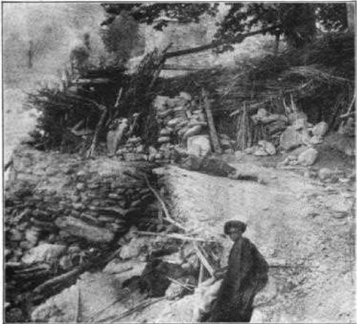
DENOLISHED SUMMER-HOUSE WITH LOWER PART OF THE GUN TOWER IN THE BACKGROUND.
